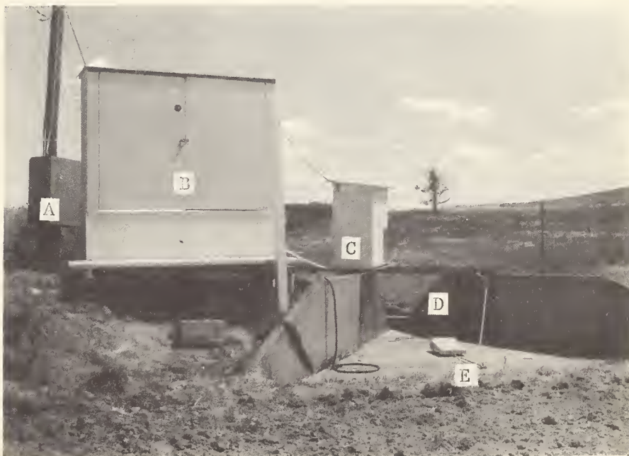
Figure 13.--Runoff measuring and sampling installation, looking downhill from experimental watershed: A, switchbox for electric power; B, shelter for refrigerator, sampler pump, and controls; C, shelter for water-stage recorder, and stilling well for float and mercury on-off switch; D, runoff rate measuring flume; E, intake sampling tube; F, purge discharge line from pump.
